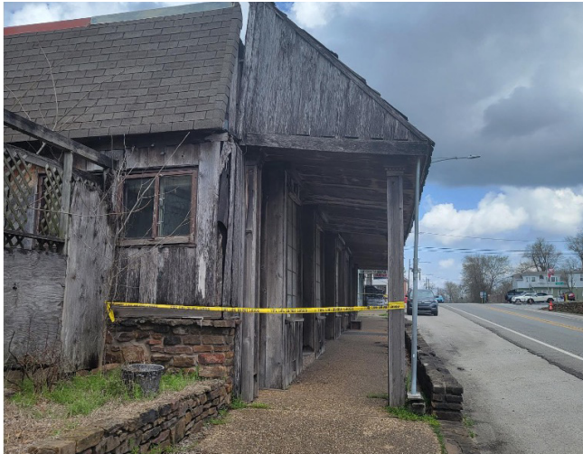
The sidewalk along this Main Street building is unsafe, due to the awning pulling away from the building's facade.
