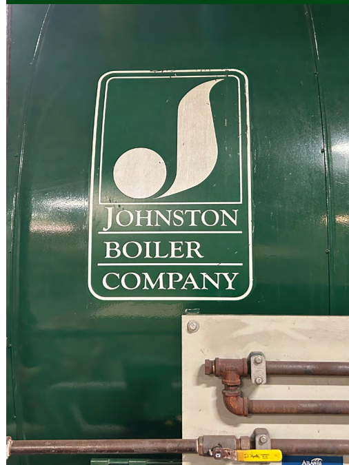
The boilers in Penn South's co-gen plant generate significant power and heat for the co-op.
