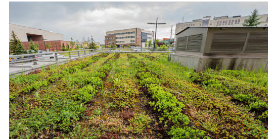
Solar arrays, white roofing material, and green roofs can make good use of wide flat roofing surfaces to capture energy, reflect the sun’s rays, or to help mitigate rain water.
