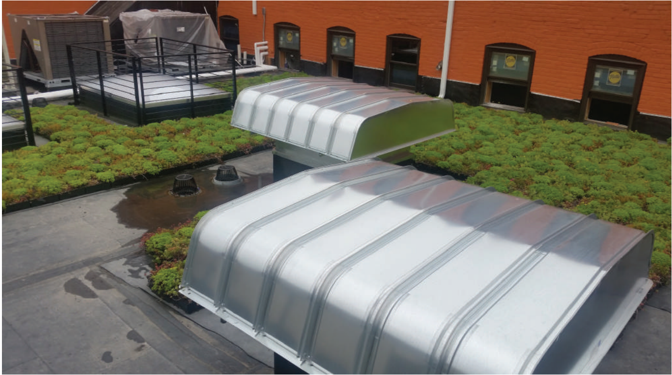
Green roof on historic restoration in New Center district, Detroit (Trisha White)
