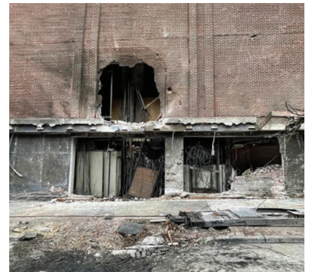
The blast site shows significant damage, specifically to an AT&T substation building.
