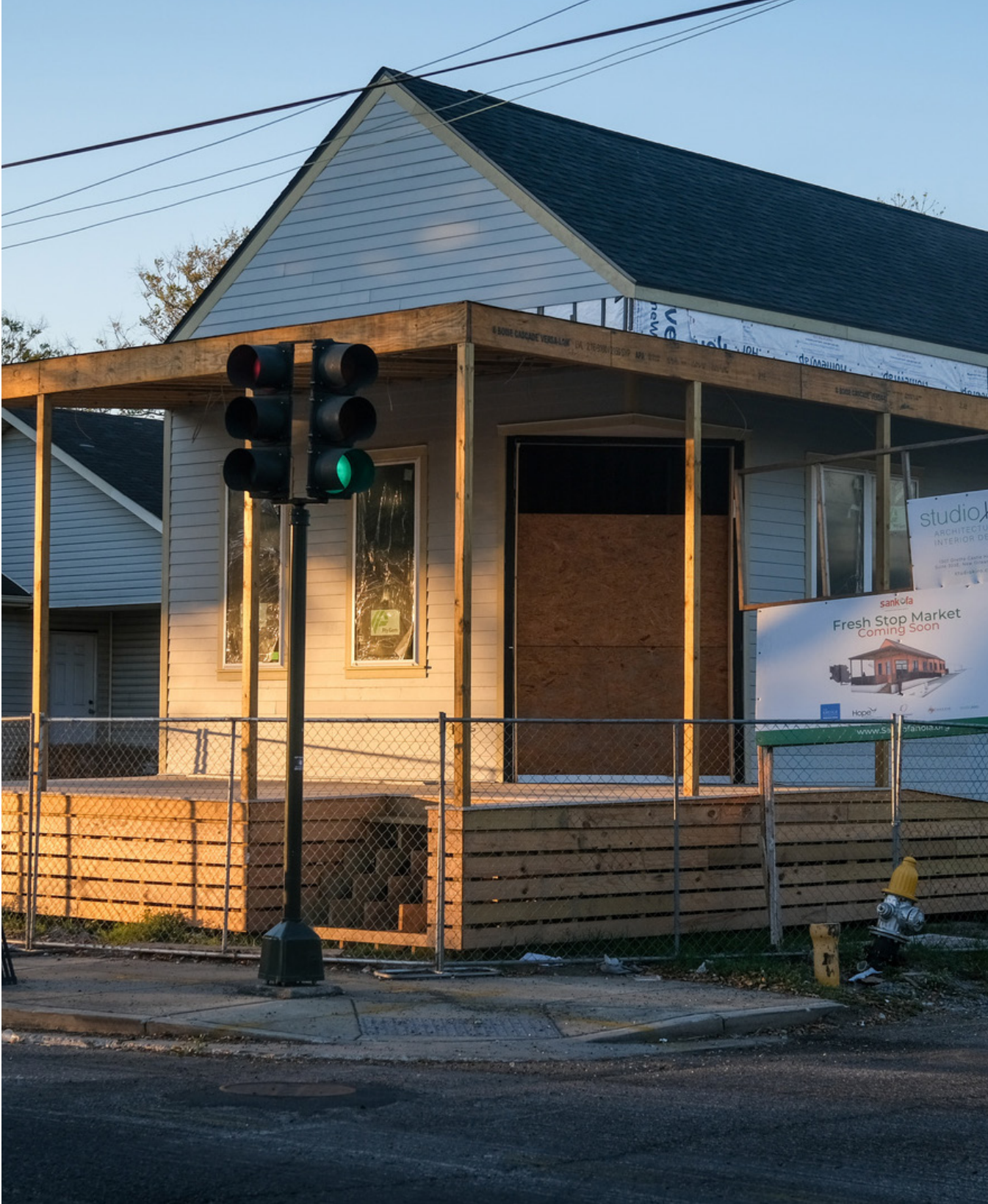
The Fresh Stop Market, a commercial endeavor by Sankofa Community Development Corporation, is under construction and will soon provide the neighborhood with proximate, if somewhat limited, grocery access.
