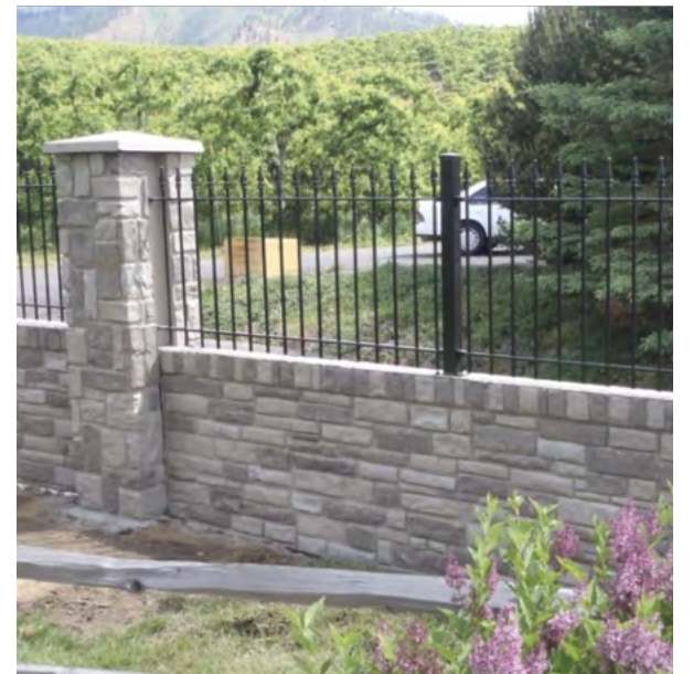
(top) The current fence around the shopping center perimeter is bent and broken in places. (bottom) The panel recommends a replacement fence employ both masonry, to act as a barrier, and metal slats for visibility.
