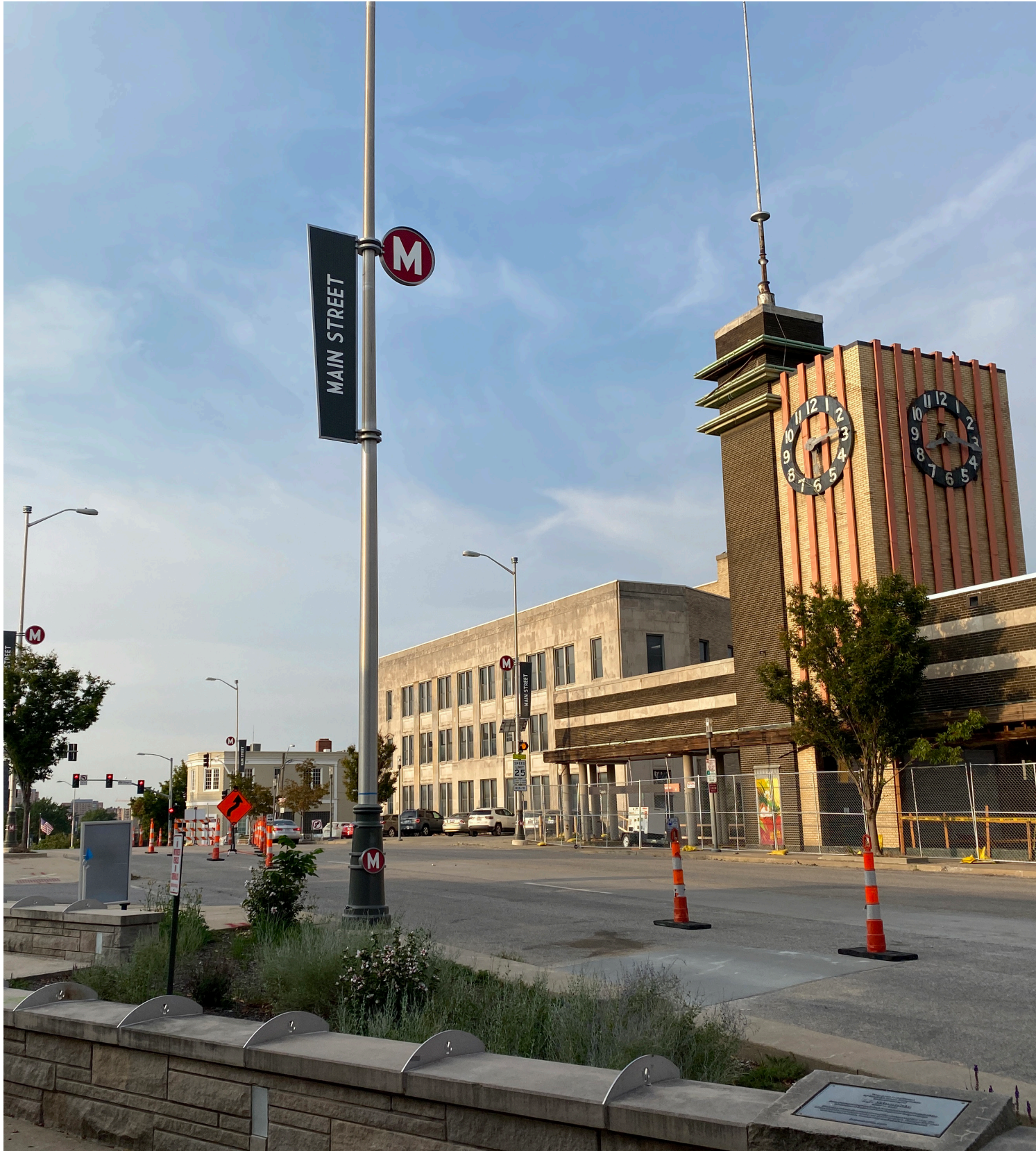
In addition to construction along the streetcar extension infrastructure, there are a number of buildings under renovation along Main Street.
