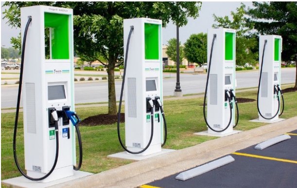
Electrical supply and vehicle infrastructure.
