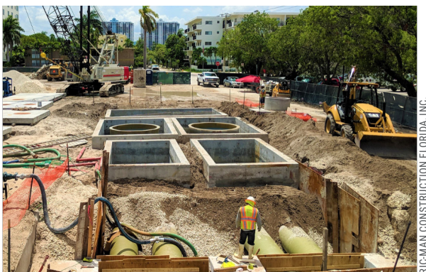
This Miami, Florida, pump station is a good example of grey infrastructure for sea level rise management.
