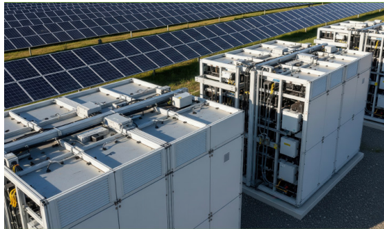
Renewable Energy + Battery Storage + Microgrid
