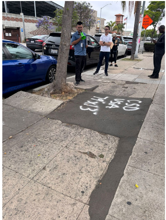
Sidewalk damaged from tree roots.
