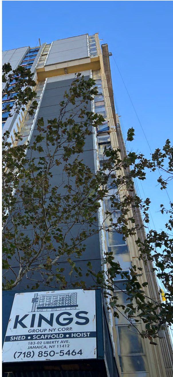
Under renovation, the Kingsbury Towers will deliver additional residential options to downtown Trenton.
