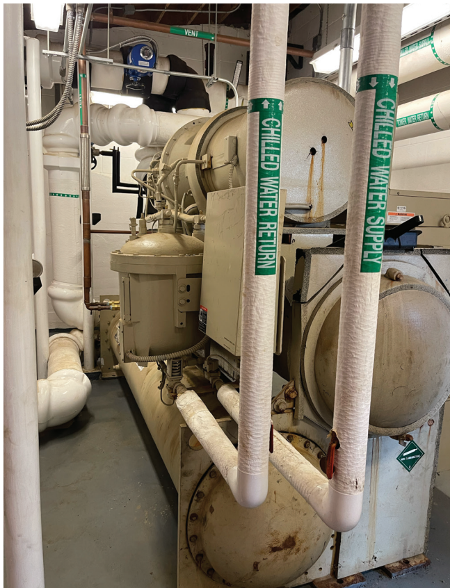
Mechanical room in Founders Hall.
