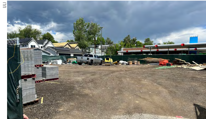
The former city hall site is being used temporarily to stage construction materials.
