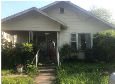
DISTRESSED SINGLE FAMILY HOME
