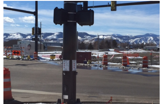
Station area features spectacular views and active industrial uses but a lack of safe and inviting pedestrian and bike amenities.
