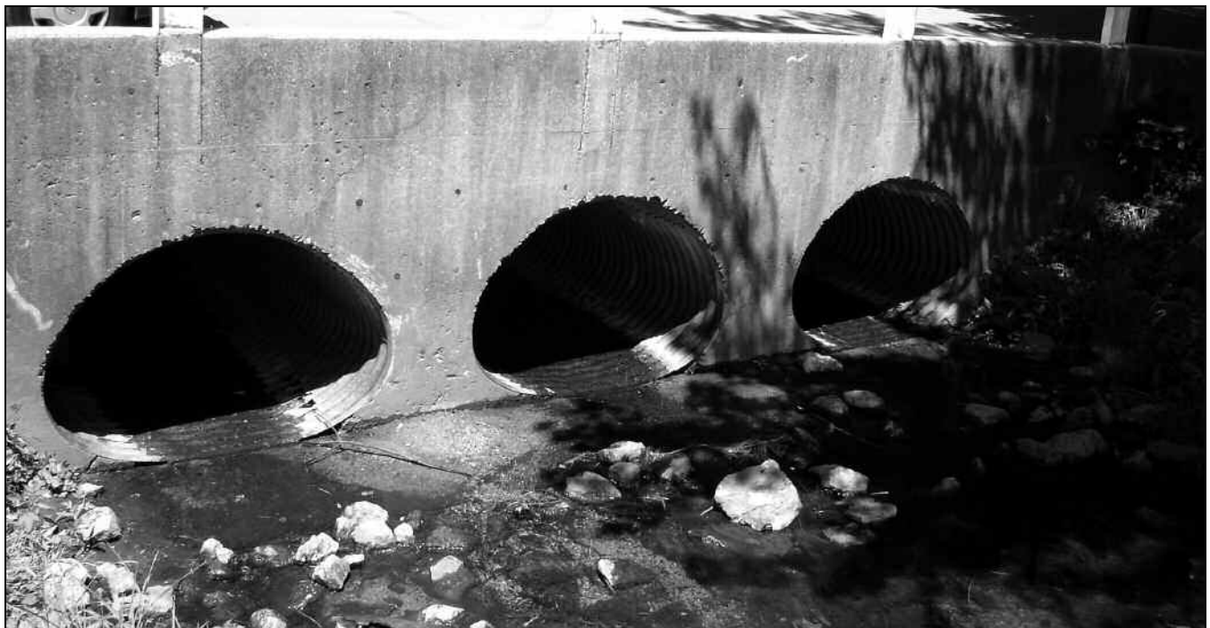
Figures 9 Heavy engineering solutions reduce the water quality and attractiveness of natural waterways.
