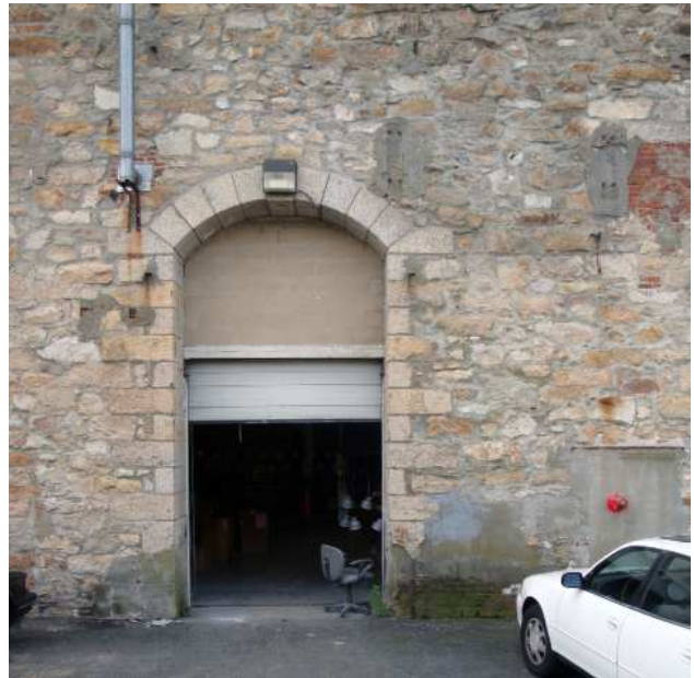
The renovated historic stonework of this mill building—the Fall River Bleachery, constructed in 1872 and added to the National Register of Historic Places in 1983—reflects Fall River's industrial roots.
