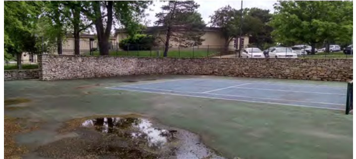
Storm Water Damaged to Tennis Court
